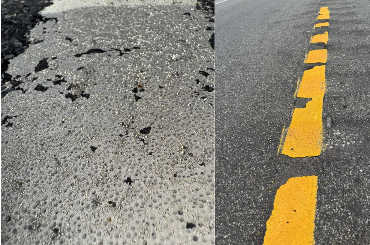
Figure 23. Images of Markings with Damage.
